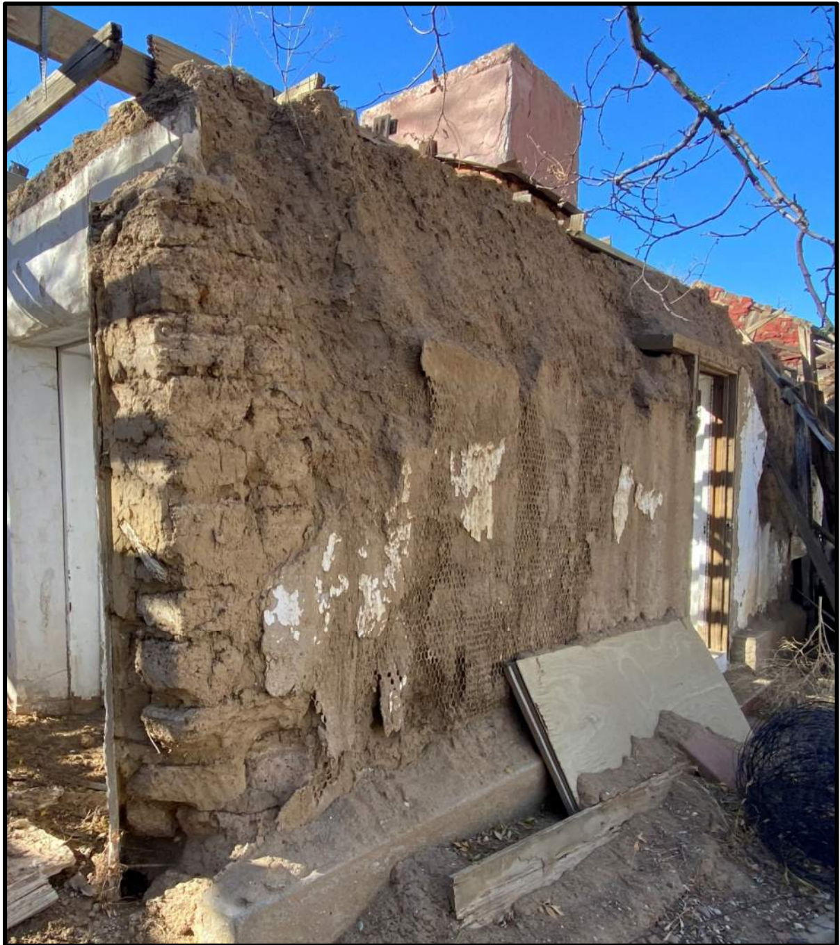
Disintegration of Adobe at Original 1850s Structure
